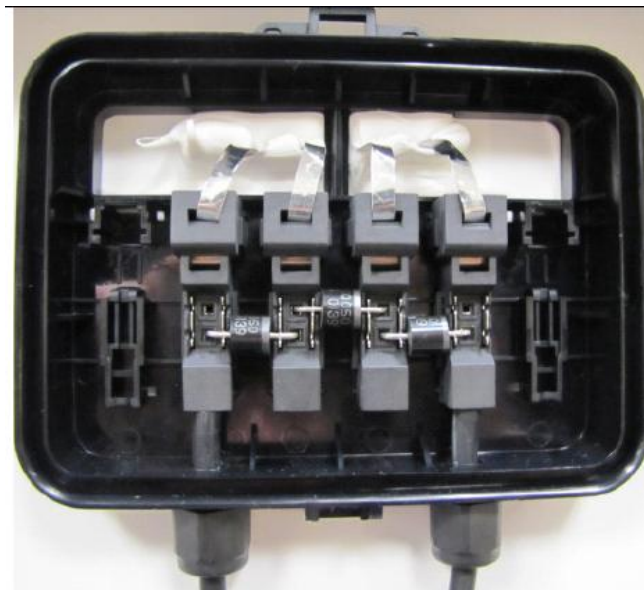
Junction box of sample 1
